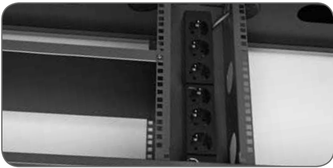
Space for power socket
